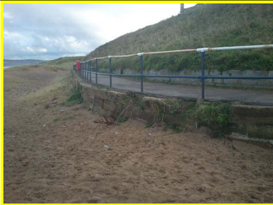
Missing coping blocks on wall below path. (Asset Ref No 12221C901C0702C03)
