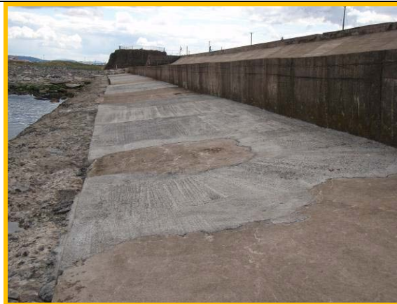
Slab repairs to deck on east side of structure – 2010 (Asset Ref No 12221C901C0506C01)
