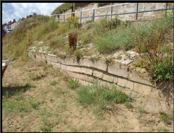
Local settlement of masonry structure (Asset Ref No 12221C901C0702C02) Photo from 2010 Report
