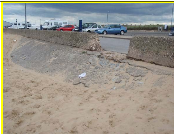
Gap in concrete wall and exposed revetment Photo from 2010
