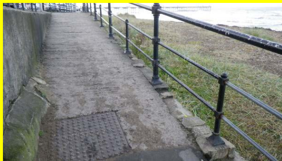
Missing coping stones to edge of path (Asset Ref No 1221C901C0704C06)
