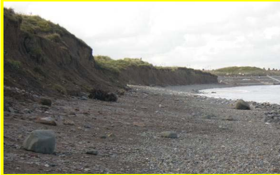
E52/10 Interface between new seawall and cliff at Mill Howle (Locally Active)
