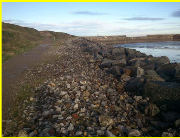
View of crest infill rubble adjacent to path has been scattered by wave overtopping (Asset Ref No. 1221D901D0202C01)
