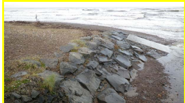
Armouring at edge of outfall from Skelton Beck (Asset Ref No 1221C901C0704C06)
