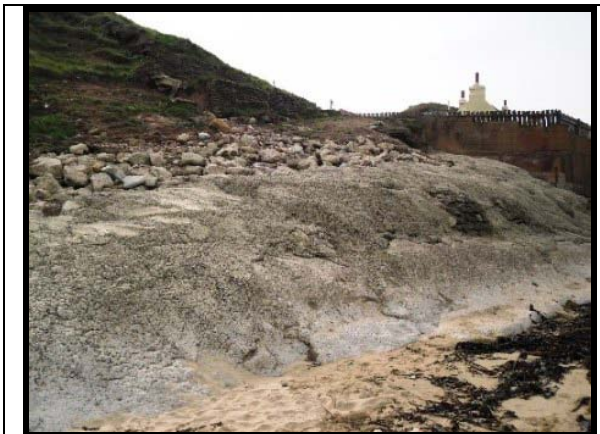
Undercutting and excavation of concrete defences (Asset Ref No. 1221C901C0704C05) Photo from 2010
