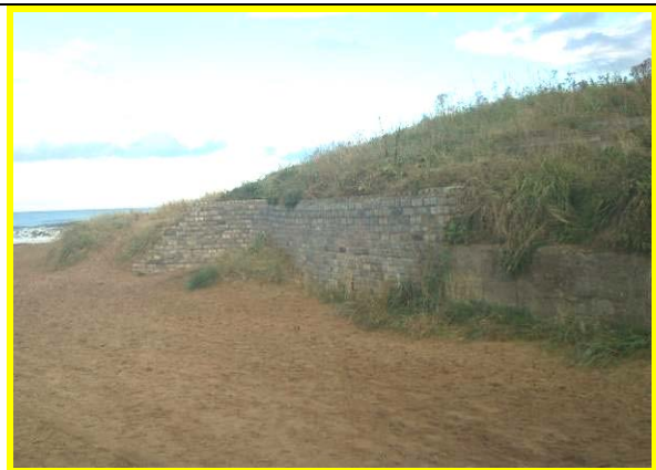
Missing masonry at seaward end of wall to southeast of beach access. (Asset Ref No 12221C901C0702C01)
