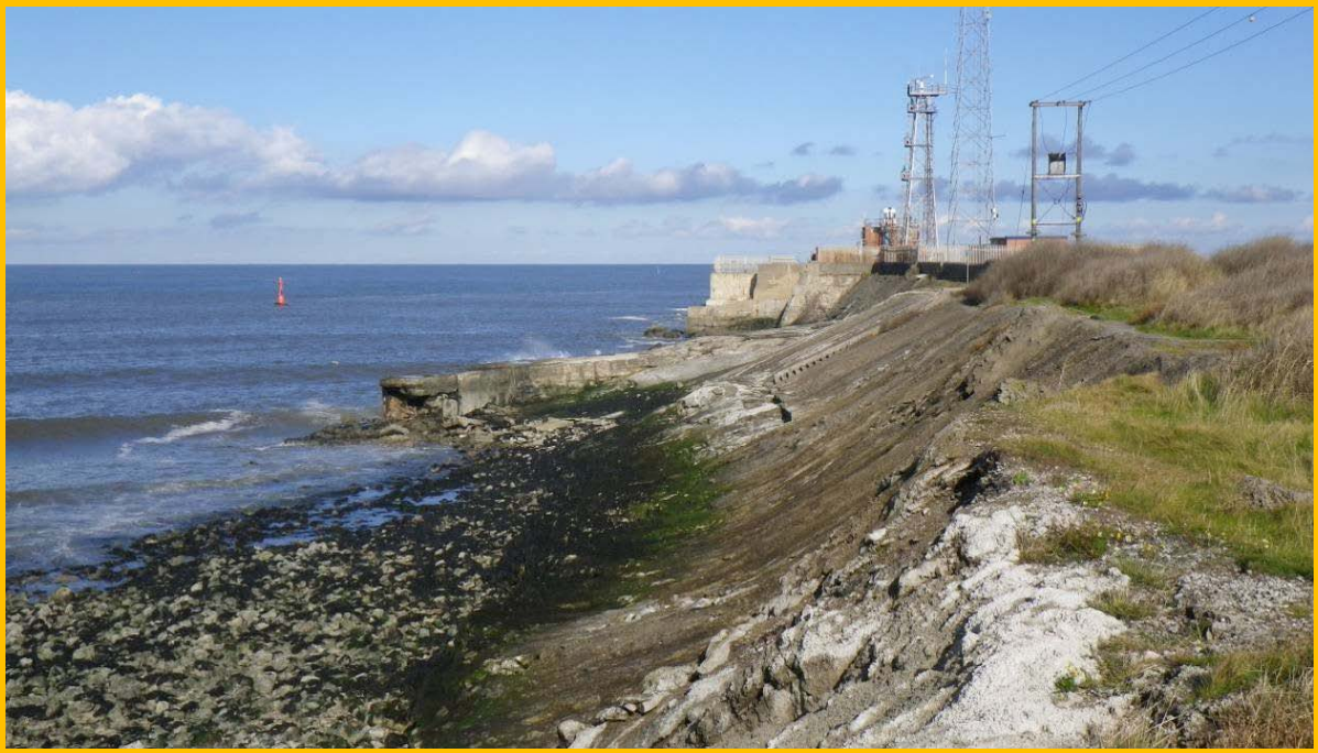
Patchwork of repairs on west side of South Gare Breakwater, recent repairs to concrete grouted revetment in foreground (Asset Ref No 12221C901C0506C01)
