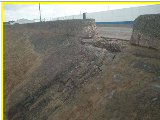
Gap in concrete wall with adjacent beach erosion from drainage, October 2012 (Asset Ref No 12221C901C0601C01)
