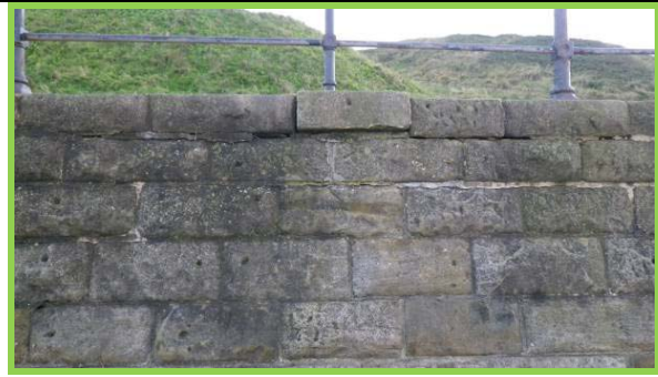
Damaged section of coping at handrail upstand (Asset Ref No 1221C901C0704C04)
