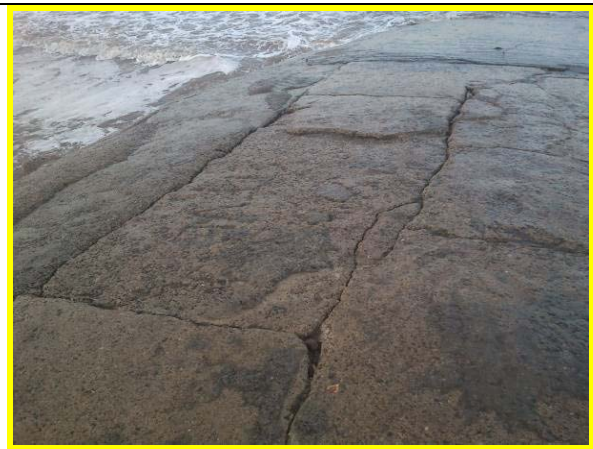
Damage to slipway at east end of Asset Ref No 1221C901C0704C03
