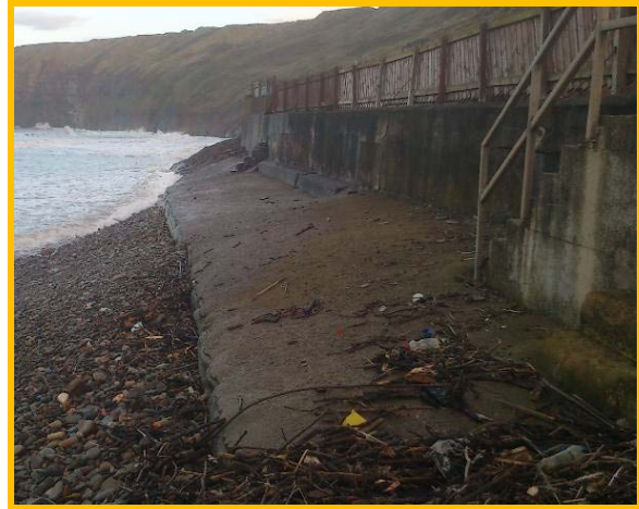
2012: Some accretion of cobbles, defence in similar condition to 2010 (Asset Ref No. 1221C901C0704C05)
