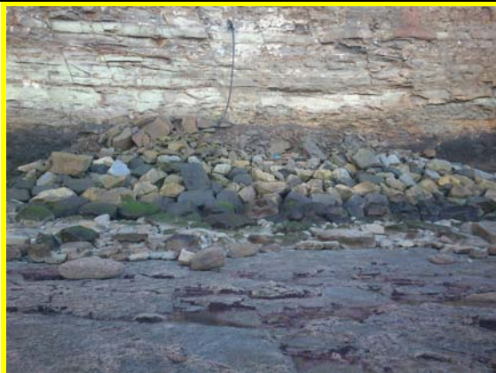
Eastern section of rock armour at cliff toe next to Cowbar lane (Asset Ref No. 1221D901D0401C01)
