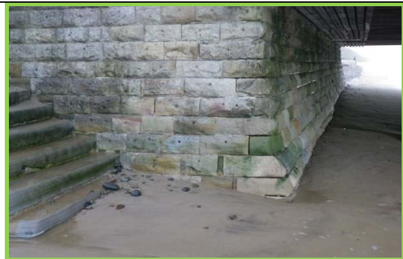
Open joints in pier abutment masonry requires repair. (Asset Ref No 1221C901C0704C04)
