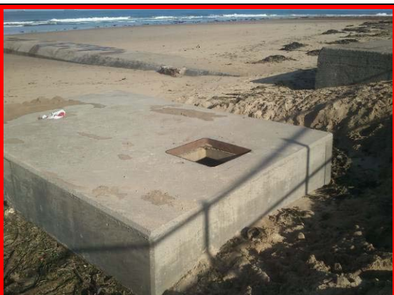
Open inspection chamber cover to west of outfall structure at Coatham beach leading to safety risk of falls into deep void / confined space. (Adjacent to asset Ref No 12221C901C0601C01)
