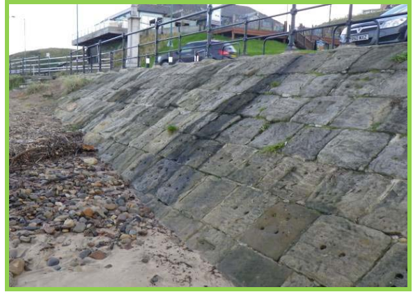
View of sloping masonry revetment at car park area. (Asset Ref No 1221C901C0704C01)
