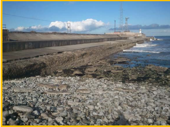
View of east side of South Gare breakwater, showing debris from failed deck slabs on beach. (Asset Ref No 12221C901C0506C01)
