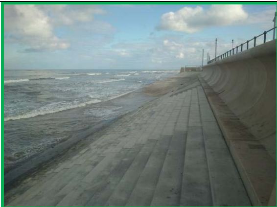
New stepped concrete seawall wall adjacent to Esplanade, Asset ref No. 1221C901C0602C02
