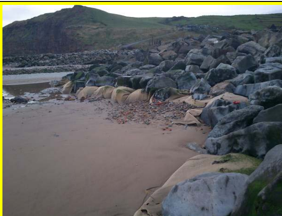
Exposed geotextile matting at rock armour toe. (Asset Ref No. 1221D901D0202C02)
