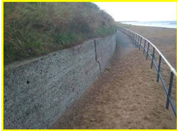
Crack in wall – photo from 15/10/2012. (Asset Ref No 12221C901C0702C03)
