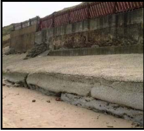
Repairs visible, but defence still shows evidence of cracking and erosion (Asset Ref No. 1221C901C0704C05) Photo from 2010
