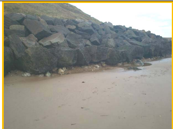
Low beach levels have exposed toe of rock armour to scour damage (Asset Ref No. 1221D901D0202C01)
