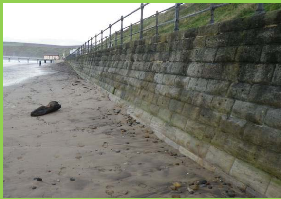
General view of wall looking south, showing abrasion near toe (Asset Ref No 1221C901C0704C04)
