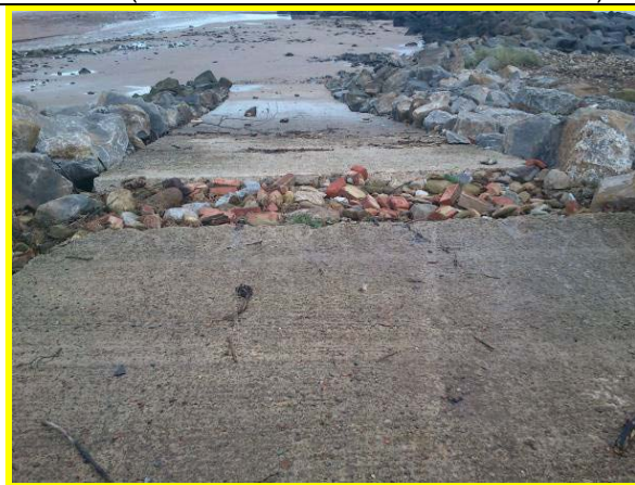
Slipway from boatpark on root of fishtail groyne showing missing section near crest filled with rubble. (Asset Ref No. 1221D901D0202C05)
