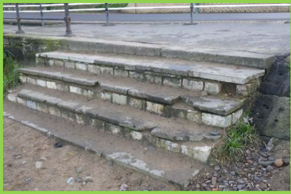
Damaged steps to beach (Asset Ref No 1221C901C0704C01)
