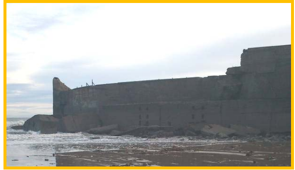
Seaward side of jetty showing failed sections and displaced slabs (Asset Ref No. 1221D901D0201C02)
