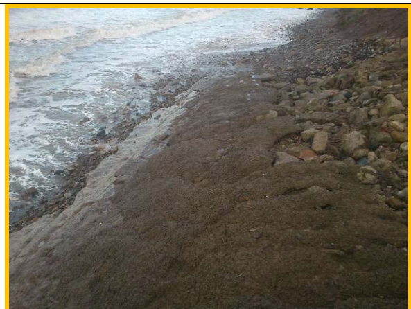
Damage to poured concrete over rubble defence. (Asset Ref No. 1221C901C0704C05)
