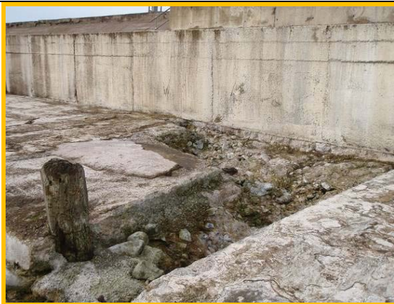
Voids present in deck - 2008 (Asset Ref No 12221C901C0506C01)
