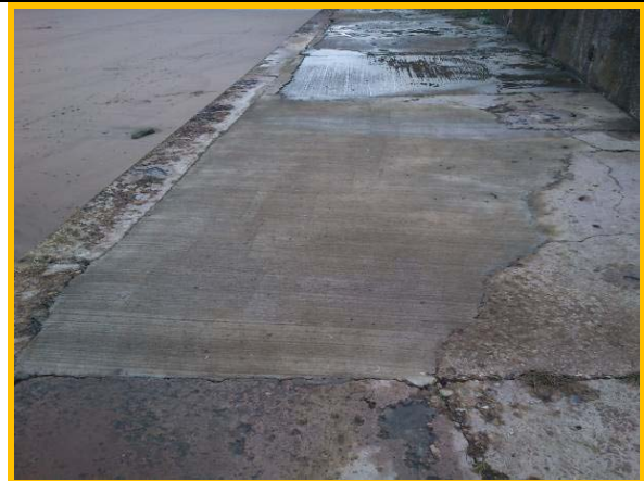
Patchwork repairs to promenade slabs. (Asset Ref No. 1221D901D0202C03)
