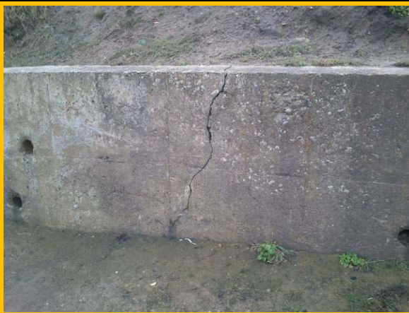
Crack in low rear retaining wall. (Asset Ref No. 1221D901D0202C03)
