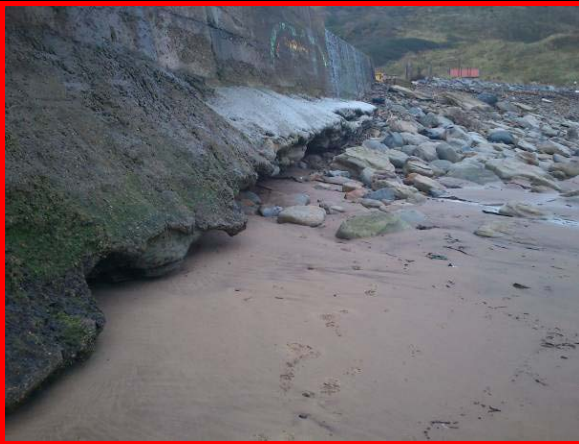
Undermining of wall toe exposing deep voids. (Asset Ref No. 1221D901D0202C03)
