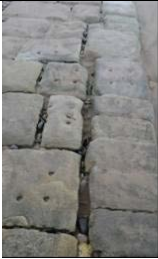
Example of area where repointing is needed to blockwork (Asset Ref No 1221C901C0704C04)
