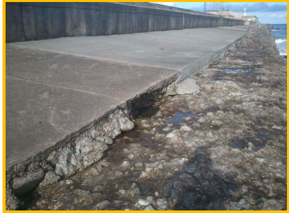
Repaired deck slabs over voids appear to be holding but facing to outer structure missing (Asset Ref No 12221C901C0506C01)
