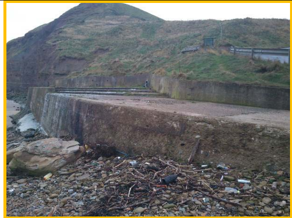
General view of wall from west end with road behind, showing eroding cliff to east in background. (Asset Ref. No 1221D901D0202C03)
